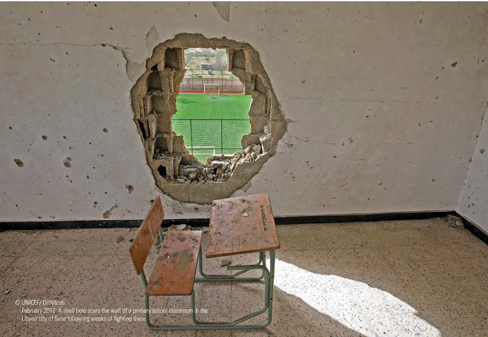
© UNICEF/Yemen April 2015: Classrooms at the Ibn Sina School in the Yemeni capital, Sana'a suffered damage during an air strike. The school, which has 1,500 girl students, is closed indefinitely.
